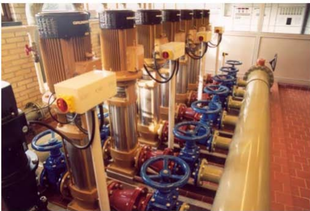
Pumps at the water works
