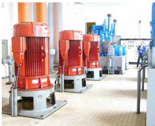
Pumping stations at the water works
